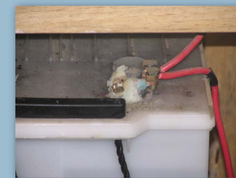
Battery only installed 6 months
